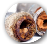
Internal Pipe Corrosion
