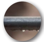
External Pipe Sweating
